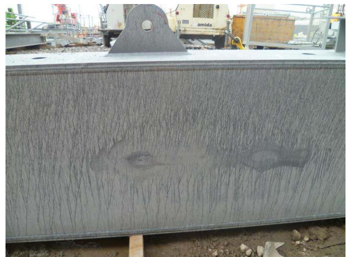
One of the beams after it rained on site showing oxide streaks
