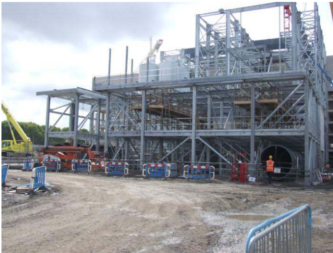
A view from the front showing the extent of the steelwork used
